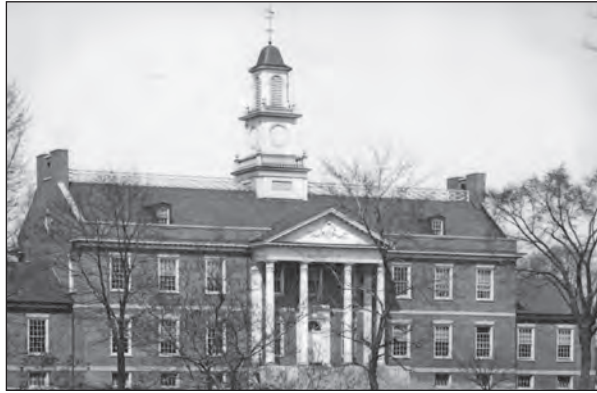
Village leaders hope to replace the roof railing and create a new patio at the Memorial Building. (Hinsdale Historical Society photo)
